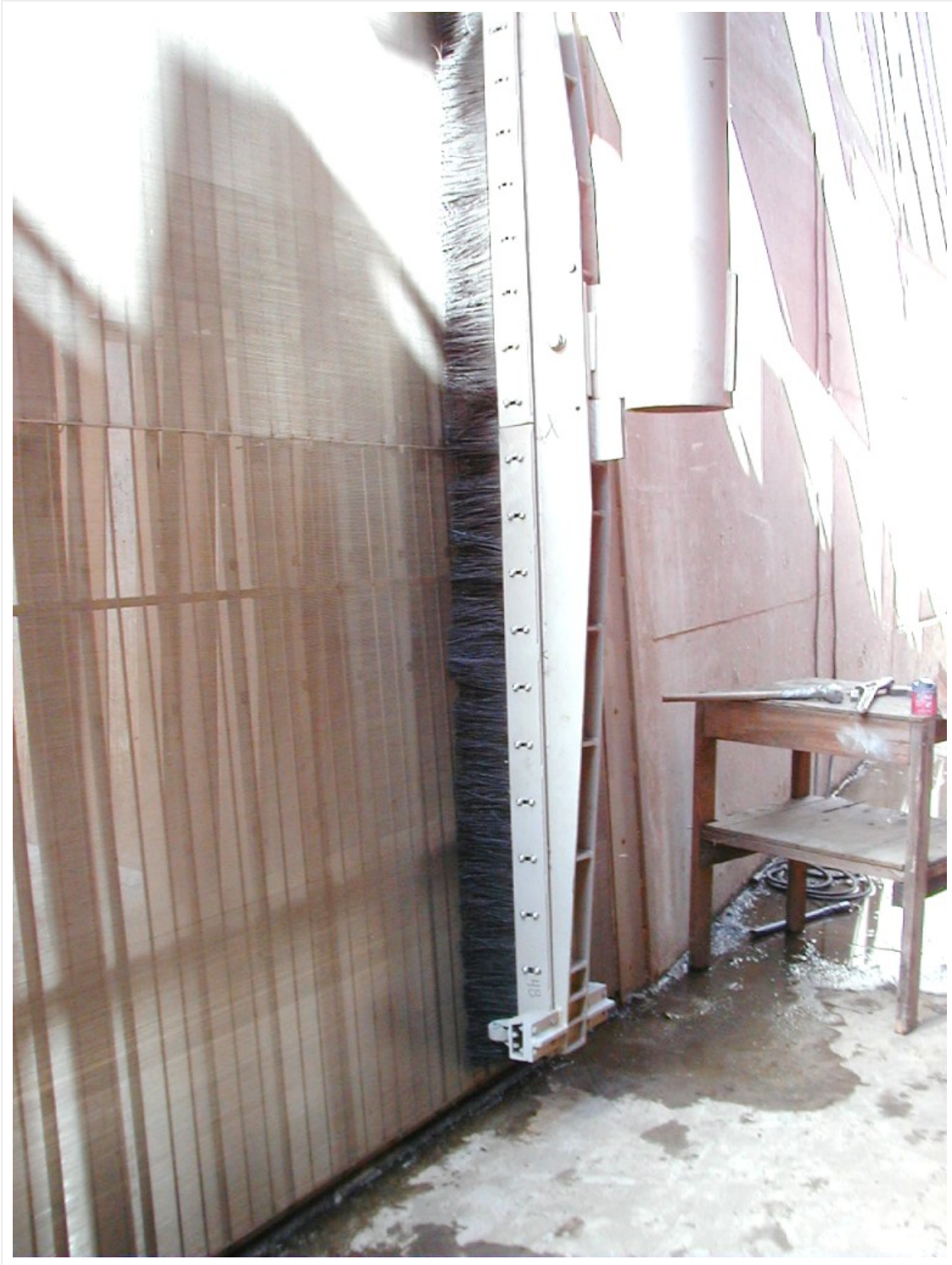
— Figure 2. Picture of a flat-plate screen wiper blade. Entire structure dewatered during construction. Picture by Dave Vogel.
