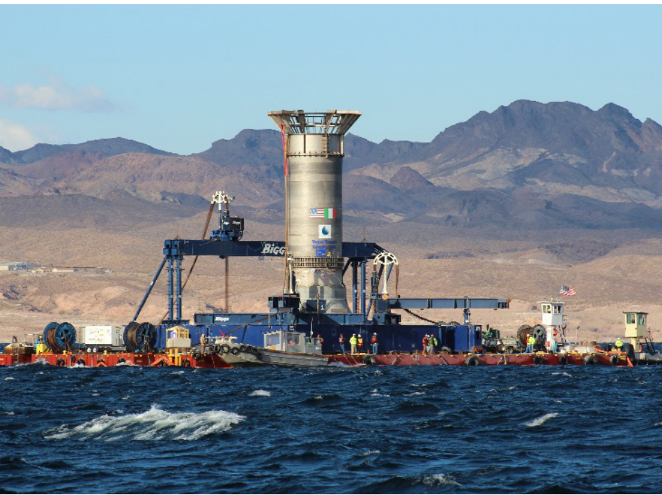
Construction of Southern Nevada Water Authority's (SNWA's) third intake at Lake Mead. The new intake structure is being floated into position via barge, to be lowered to connect to a three-mile, 20-foot diameter tunnel under Lake Mead. The $817 million intake was put into service in 2015, to allow SNWA to ensure water supplies for its customers if lake elevations drop below the level of an existing upper intake. Photo courtesy of SNWA.
