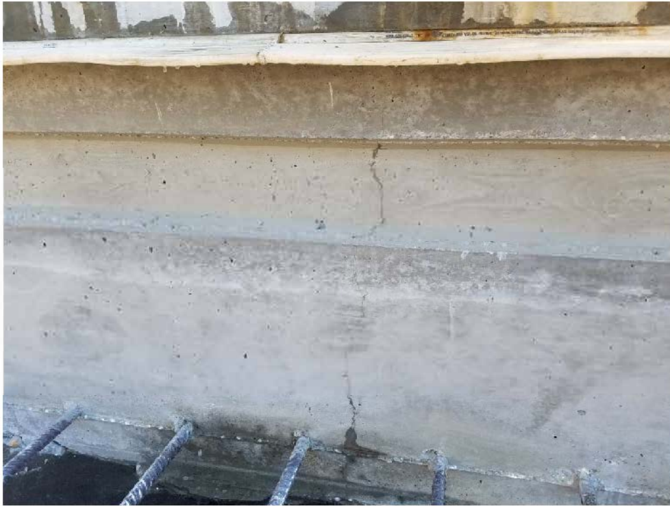
Figure 3: Typical Through Cracking Observed
