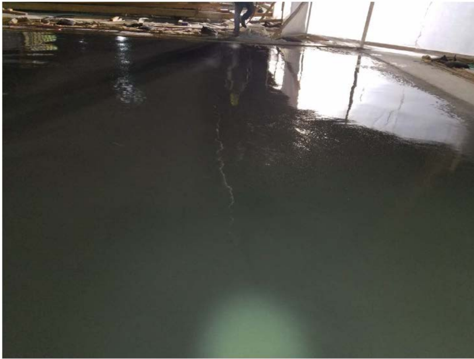
Figure 5: Cracking observed in 30C four hours after finishing
