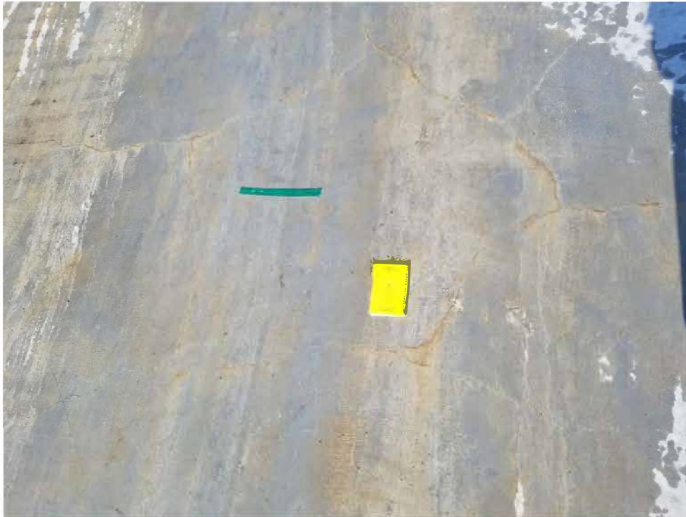
Figure 1: Typical Cracking Observed
