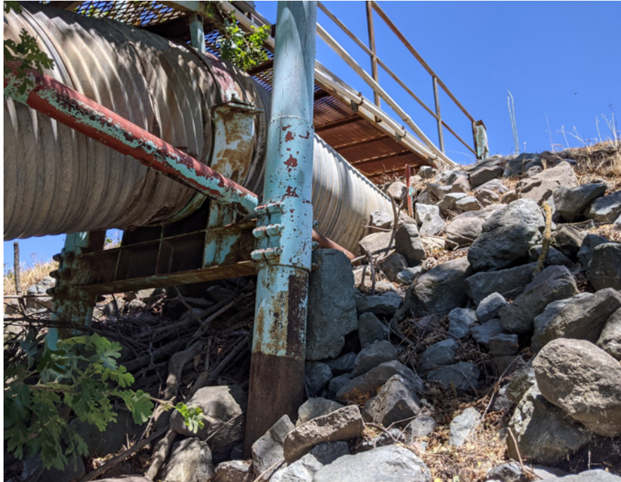
Photo 5. Removal of 36-inch corrugated metal pipe discharge pipe and where recontouring of waterside levee activities, including the placement of fabric and rip rap. Facing northeast toward levee and levee crown. December 16, 2021
