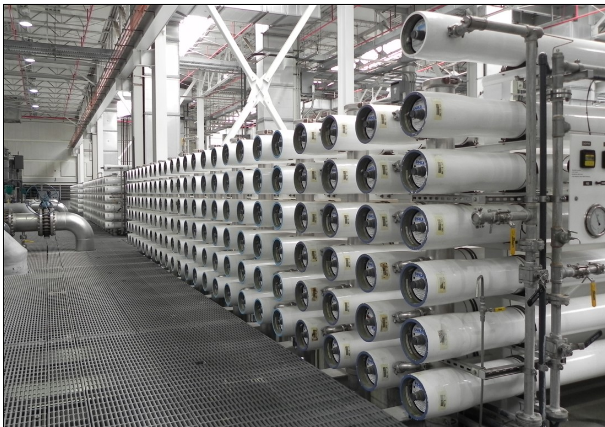
Figure 7 Reverse Osmosis at the Groundwater Replenishment System
