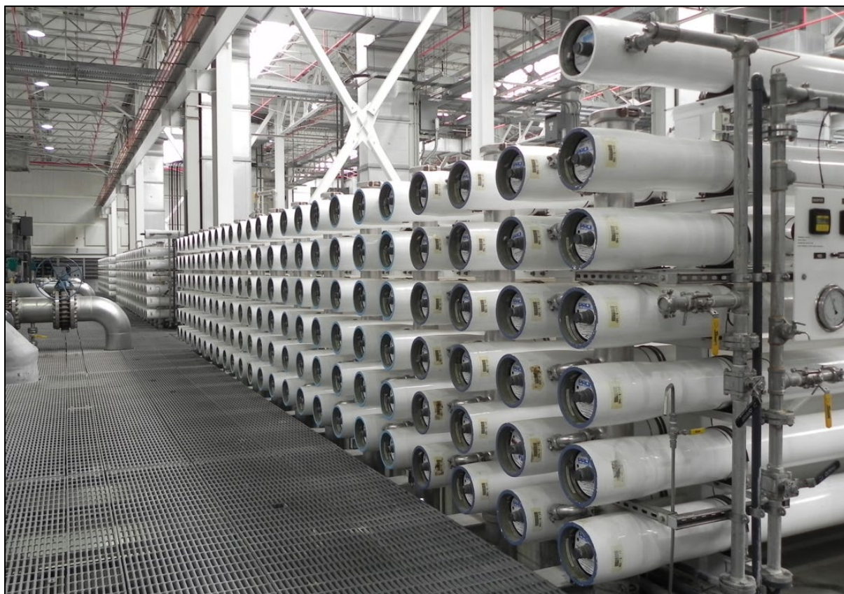
Figure 7 Reverse Osmosis at the Groundwater Replenishment System
