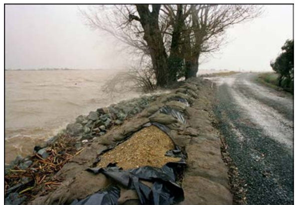
Levee damage during a storm
