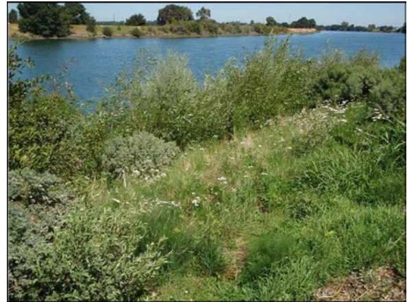
Woody and non-woody growth along base of levee
