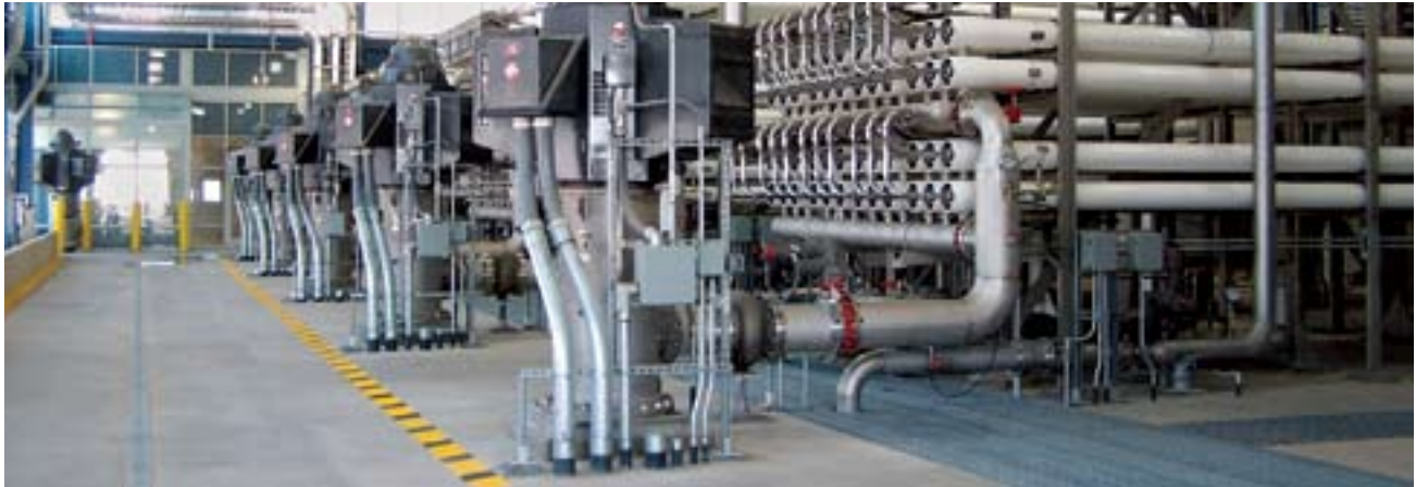
Urban water agencies are increasingly considering drought-proof water sources such as desalination for part of their water supply portfolios. In 2009 there were 29 operating desalination plants (brackish groundwater and sea water) in California.
